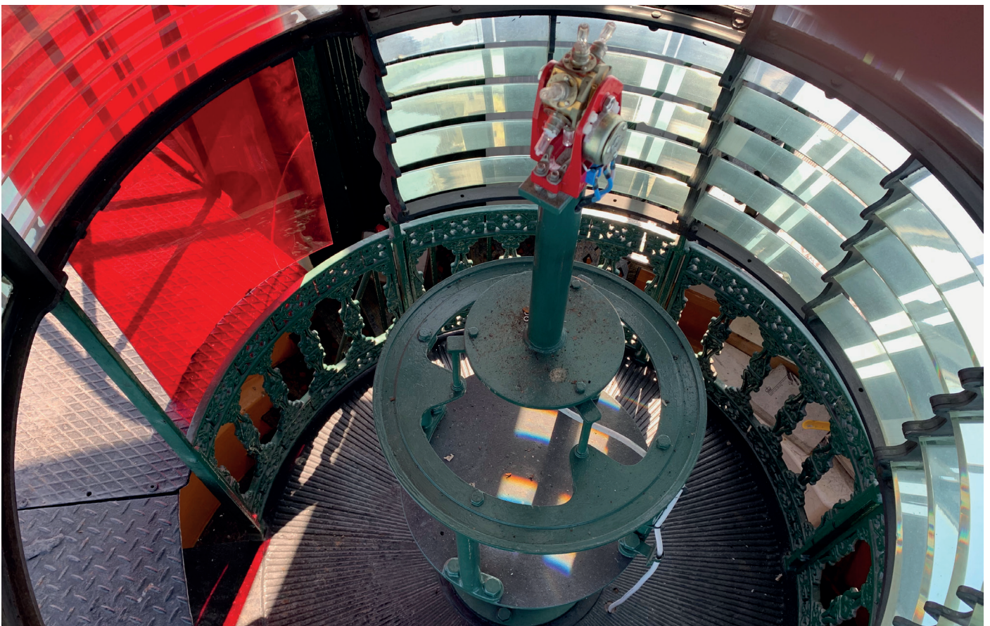
Below: In this case, there are a number of small halogen lamps that can be rotated into position if one should fail.
